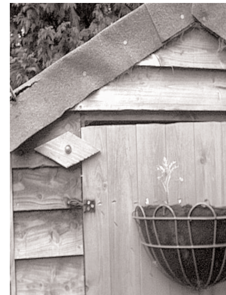
This is a fairly typical example of poor shed security!
